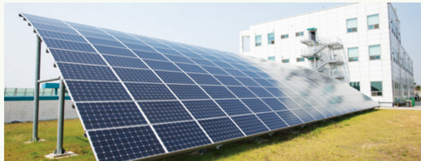
Solar Power Plant
